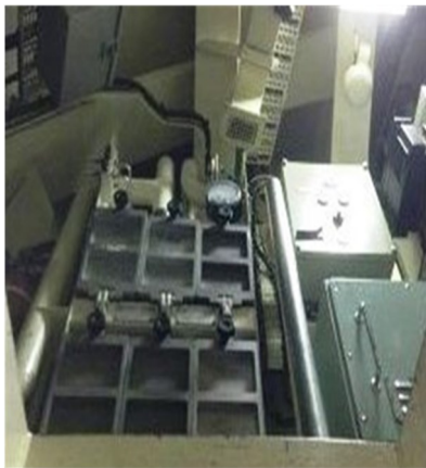
Six canisters installed in shipboard scrubber
